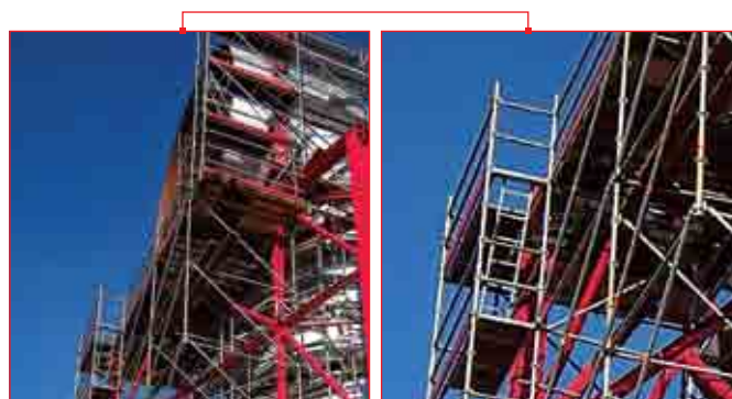
Ostrołęka Power Plant
